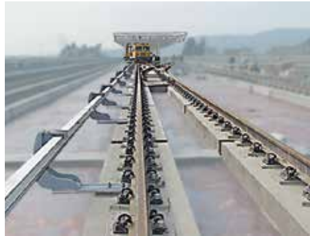
Under running 3rd rail system with glass reinforced polyester supports (Taipei)
