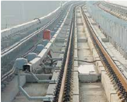
Under running 3rd rail system with fabricated steel supports
